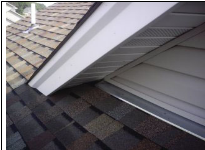
Flashing is not complete under dormer.
