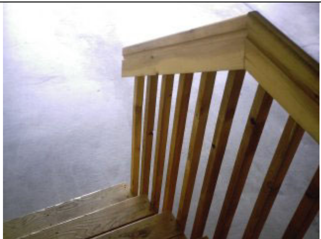
No safety graspable handrail.
