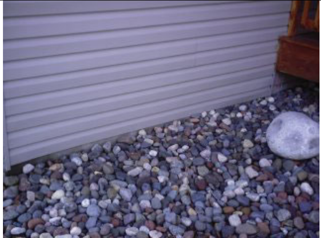
Soil too close to siding, should be 6 to 8" below.
