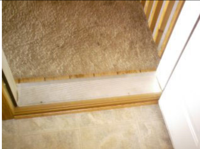
Possible trip hazards at garage/house entrance door threshold.
