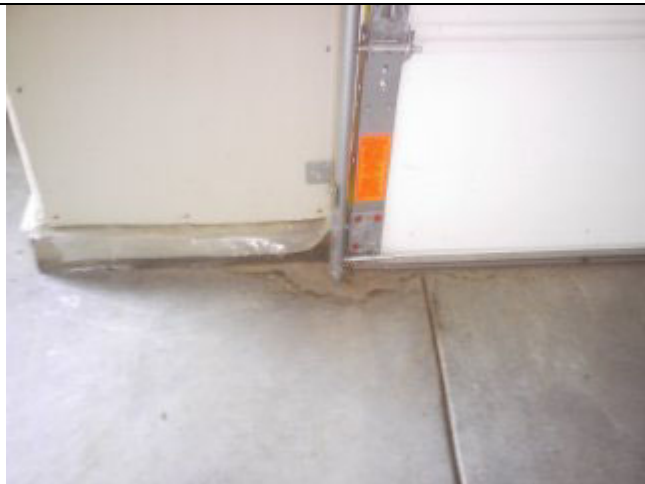
Areas where water enters around garage door.
