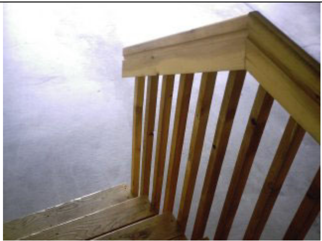
No safety graspable handrail.
