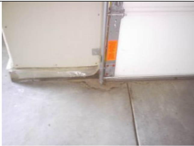
Areas where water enters around garage door.
