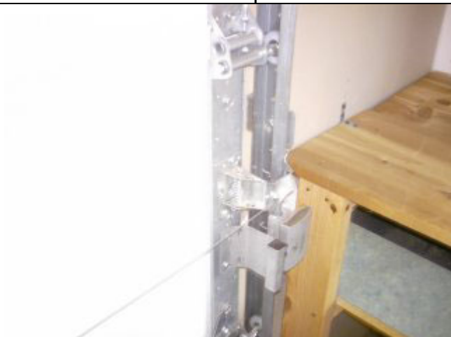
Damaged garage door lock.
