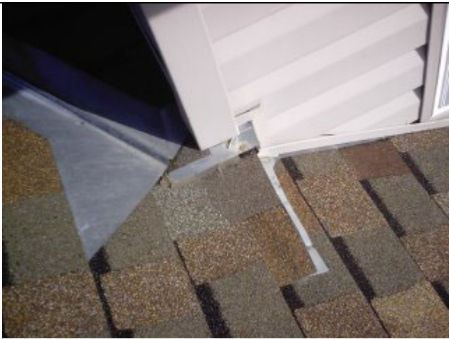
Opening in flashing.
