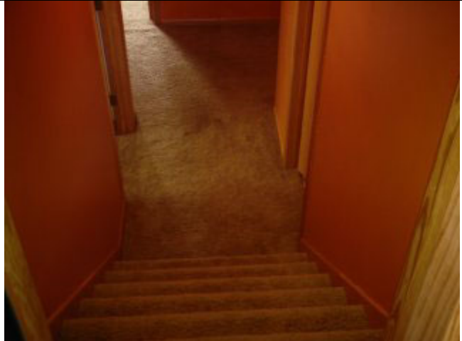
No safety handrail in hallway.
