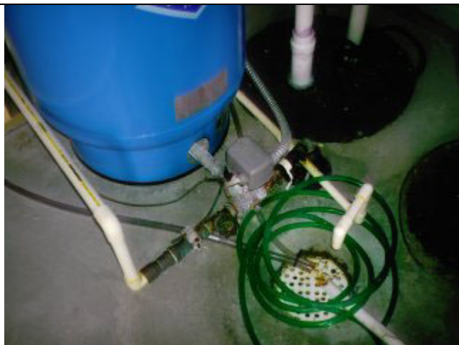
No conduit on electric supply line to switch.
