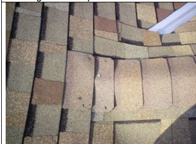
Nails are not properly set and sealed.
