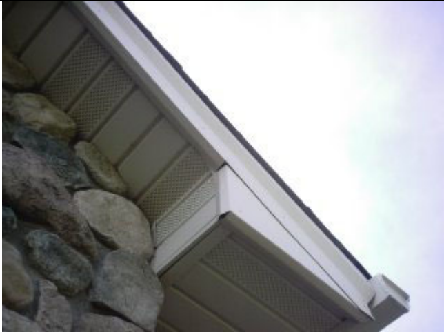
Fascia is not properly set.
