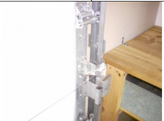
Damaged garage door lock.
