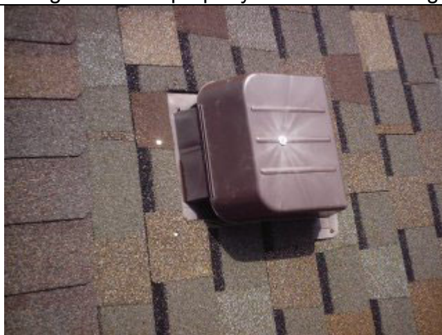
Exposed nails on roof vents.
