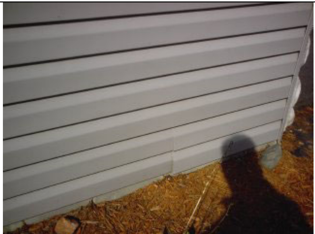
Soil too close to siding on garage, siding loose.
