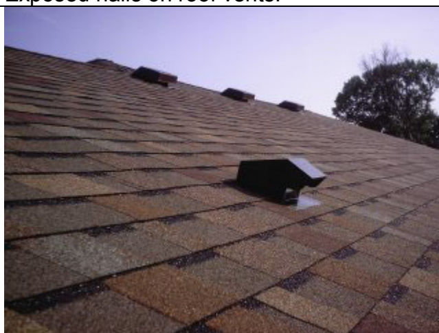
Nails are not sealed on bathroom vents.
