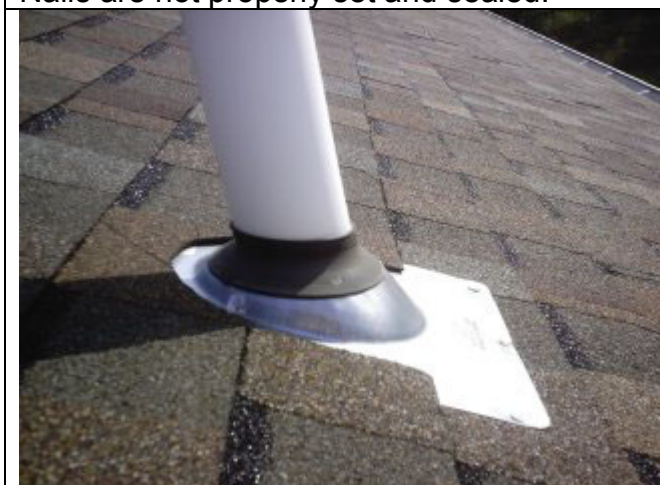
Nails are not sealed on sewer vents.
