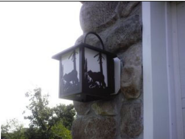
Exterior lights loose.
