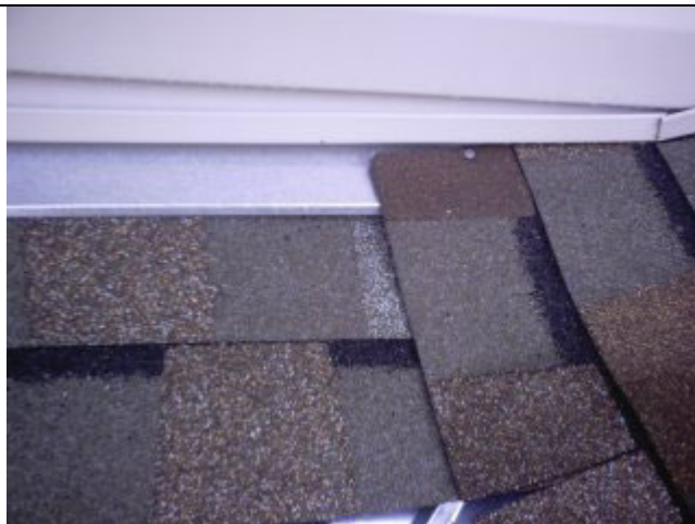
Shingles are not properly set under Flashing.
