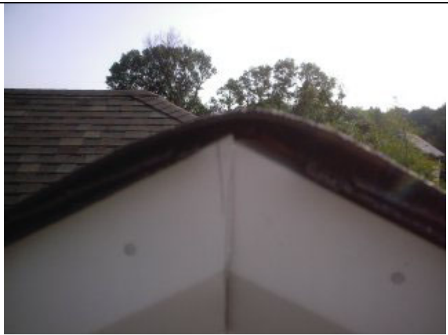
Opening in roof area at gable.
