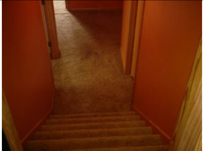
No safety handrail in hallway.
