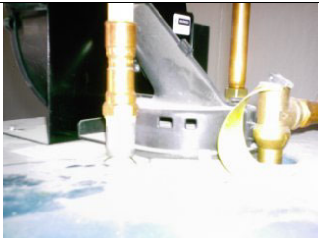
Improper connection on water heaters water supply lines between copper and steel.
